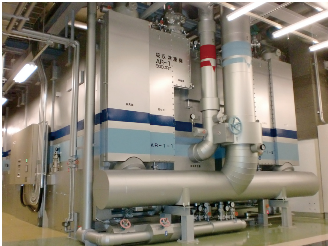
New 3,000RT absorption chiller units installed at the No2. Plant in June 2010
