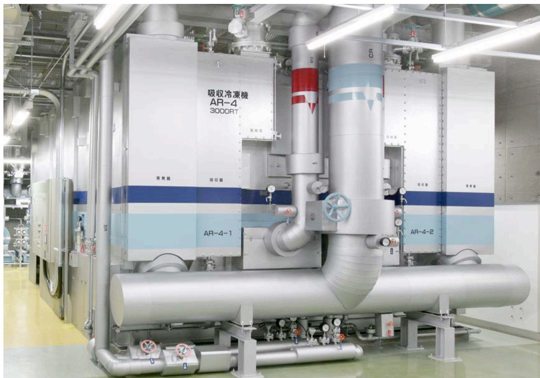
The new 3,000RT absorption chiller unit installed at the No2. Plant in June 2011
