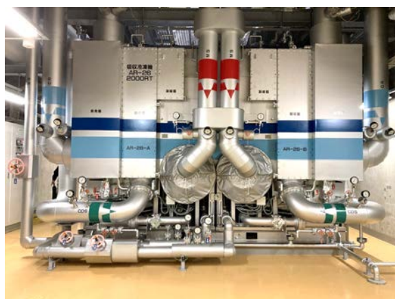
Absorption chillers (Top: 3,000RT; bottom: 2,000RT)
